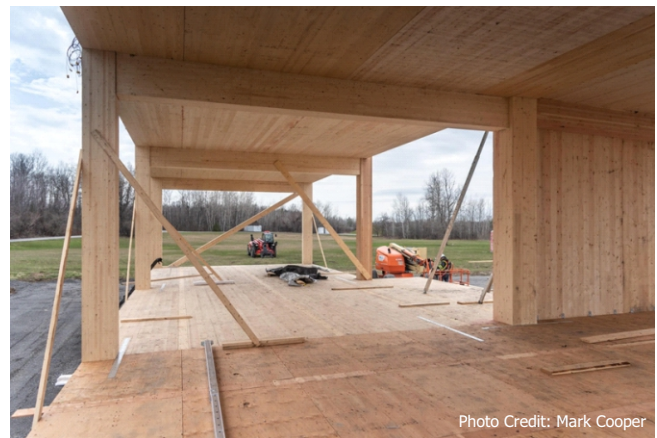
Cross-Laminated Timber, Glulam and Dowel-Laminated Timber are some of the mass timber products used in the structure.
